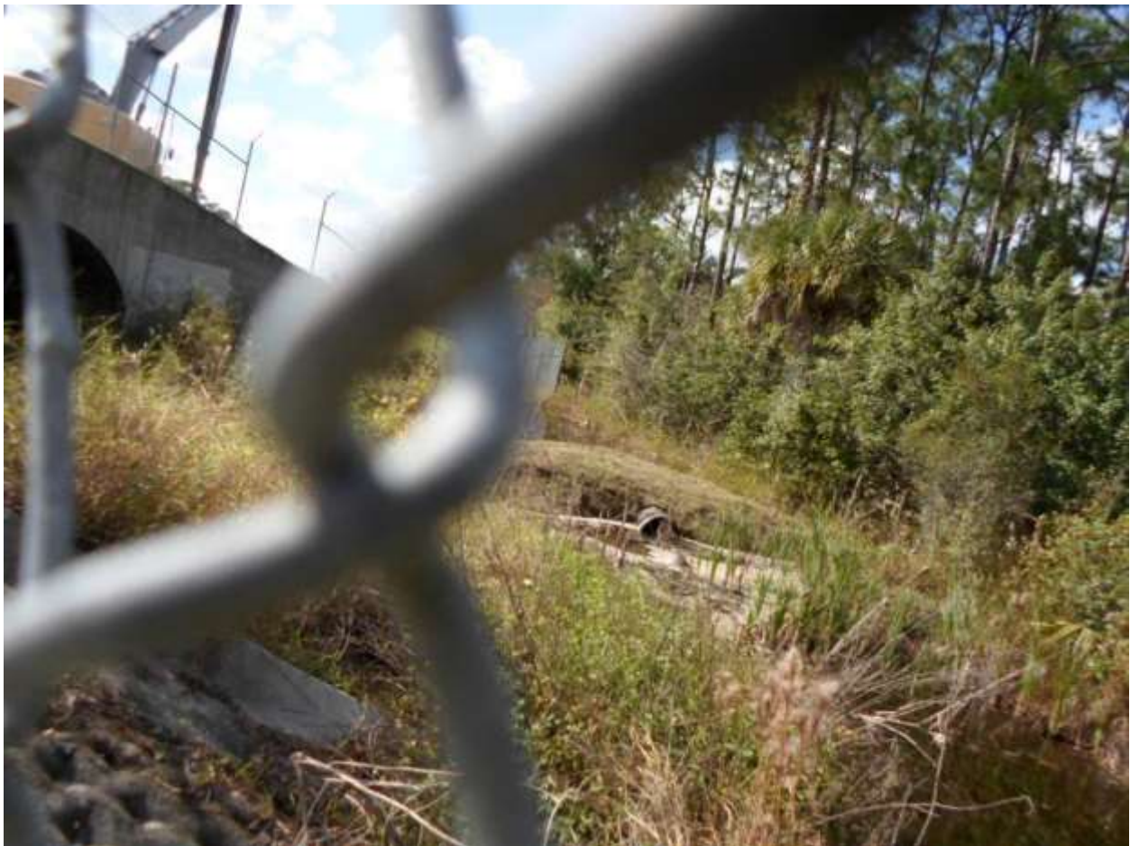
Land bridge and culvert are in the center of photo and wildlife underpass is at upper left.
