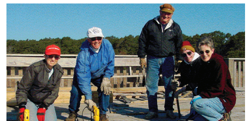
Volunteers at Chincoteague NWR (VA) reconstruct a wildlife observation platform on the refuge's marsh trail.
