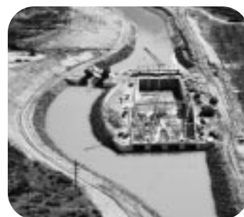
A W-SHAPED FISH SCREEN WAS INSTALLED THIS YEAR AT THE GRAND VALLEY PROJECT DIVERSION DAM AND CANAL. CANAL CHECKS BECAME OPERATIONAL IN 2002, AND A FISH PASSAGE COMPLETED IN 2005 WILL BECOME FULLY OPERATIONAL UPON COMPLETION OF THE PRICE-STUBB FISH PASSAGE IN 2007.
