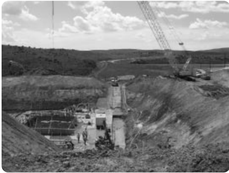
ONE OF THE FIRST MANAGEMENT ACTIONS TO OCCUR UNDER THE COOPERATIVE AGREEMENT IS THE ENLARGEMENT OF ELKHEAD RESERVOIR IN NORTHWEST COLORADO. THE RECOVERY PROGRAM IS FUNDING 5,000 ACRE-FEET OF A 12,000 ACRE-FOOT ENLARGEMENT TO MAKE WATER AVAILABLE TO AUGMENT LATE-SUMMER FLOWS IN THE YAMPA RIVER TO BENEFIT THE ENDANGERED FISH. CONSTRUCTION IS SCHEDULED FOR COMPLETION IN 2007.
