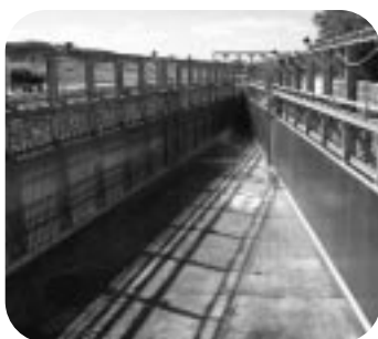
A FISH SCREEN INSTALLED AT THE REDLANDS WATER AND POWER COMPANY DIVERSION DAM AND CANAL BECAME OPERATIONAL IN 2005. THE FISH PASSAGE BECAME OPERATIONAL IN 1996.
