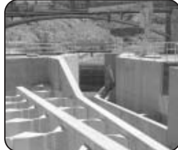
Fish passage at Grand Valley Project diversion dam.
