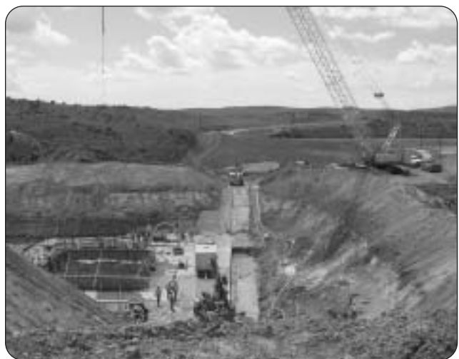
A 12,000 acre-foot enlargement of Elkhead Reservoir in northwest Colorado is underway. When completed in 2007, 5,000 acre-feet of permanent water and up to 2,000 acre-feet of leased water per year will be available to augment late-summer flows in the Yampa River.
