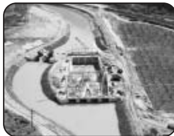
Fish screen under construction at the Grand Valley Project diversion dam and canal.
