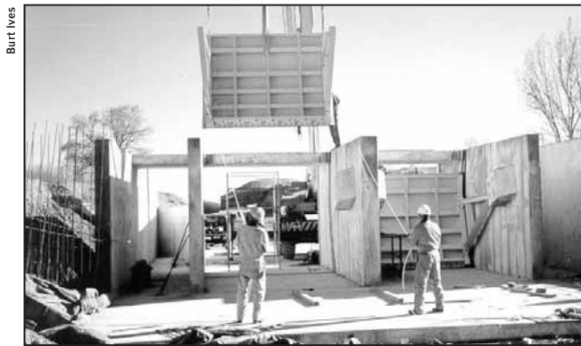
Automated gate control equipment installed at the Government Highline Canal in 2002 improved efficiency and will provide about 28,000 acre-feet of water for endangered fish.
