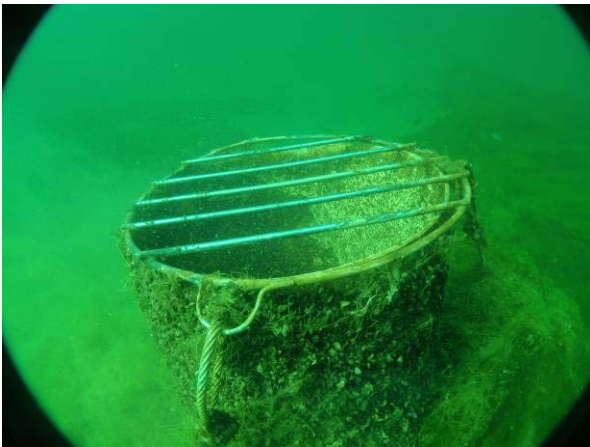
The intake for Willow Beach NFH's water supply, after being cleared of aquatic vegetation.
