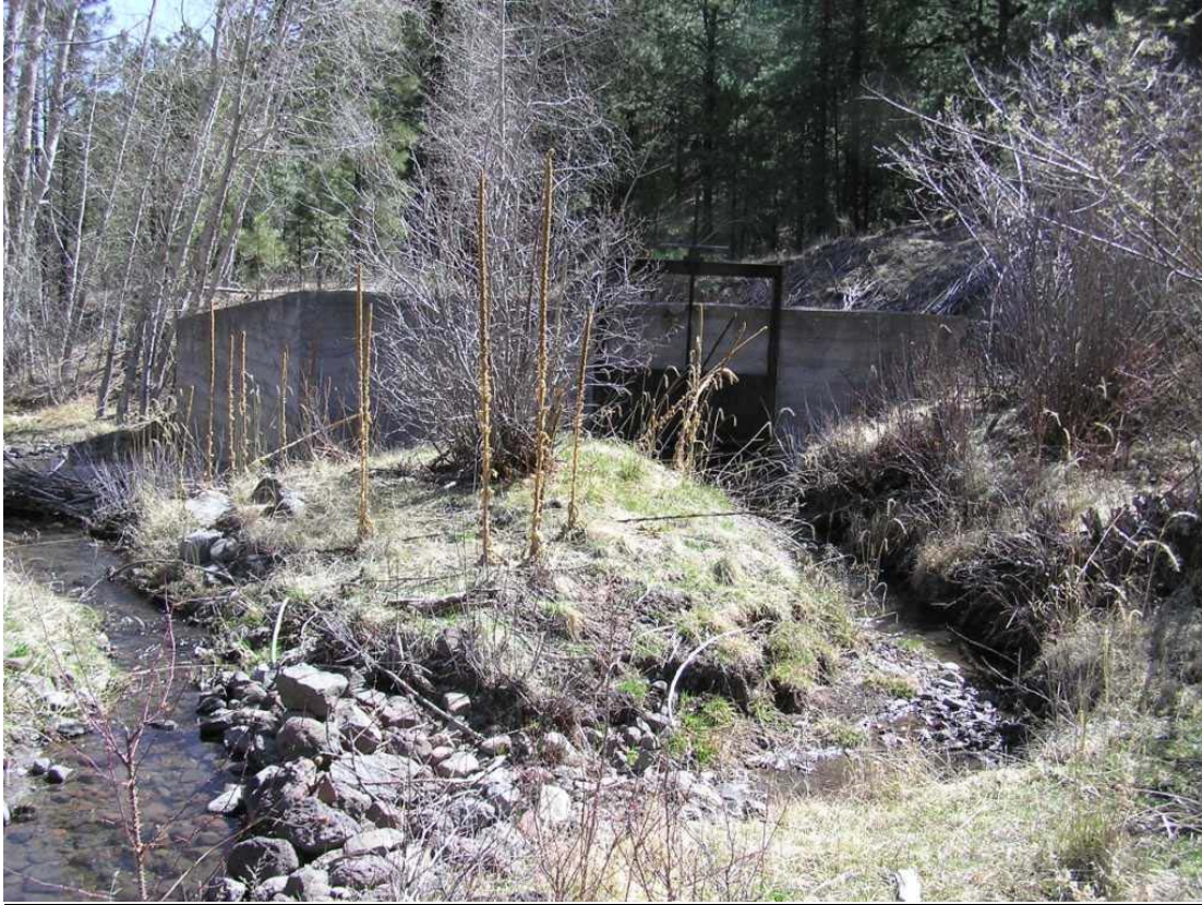
Photo 1. Downstream view from above the Rudd Creek Diversion located on the ASNF. The turnstile and irrigation channel bypass is located on the right. Water flows for a majority of the time through the concrete bypass on the left.
