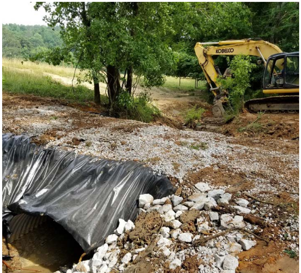
After: Newly installed 8-foot culvert allows aquatic and terrestrial passage (fencing to exclude livestock was added later). Credit: Vance Crain/SARP
