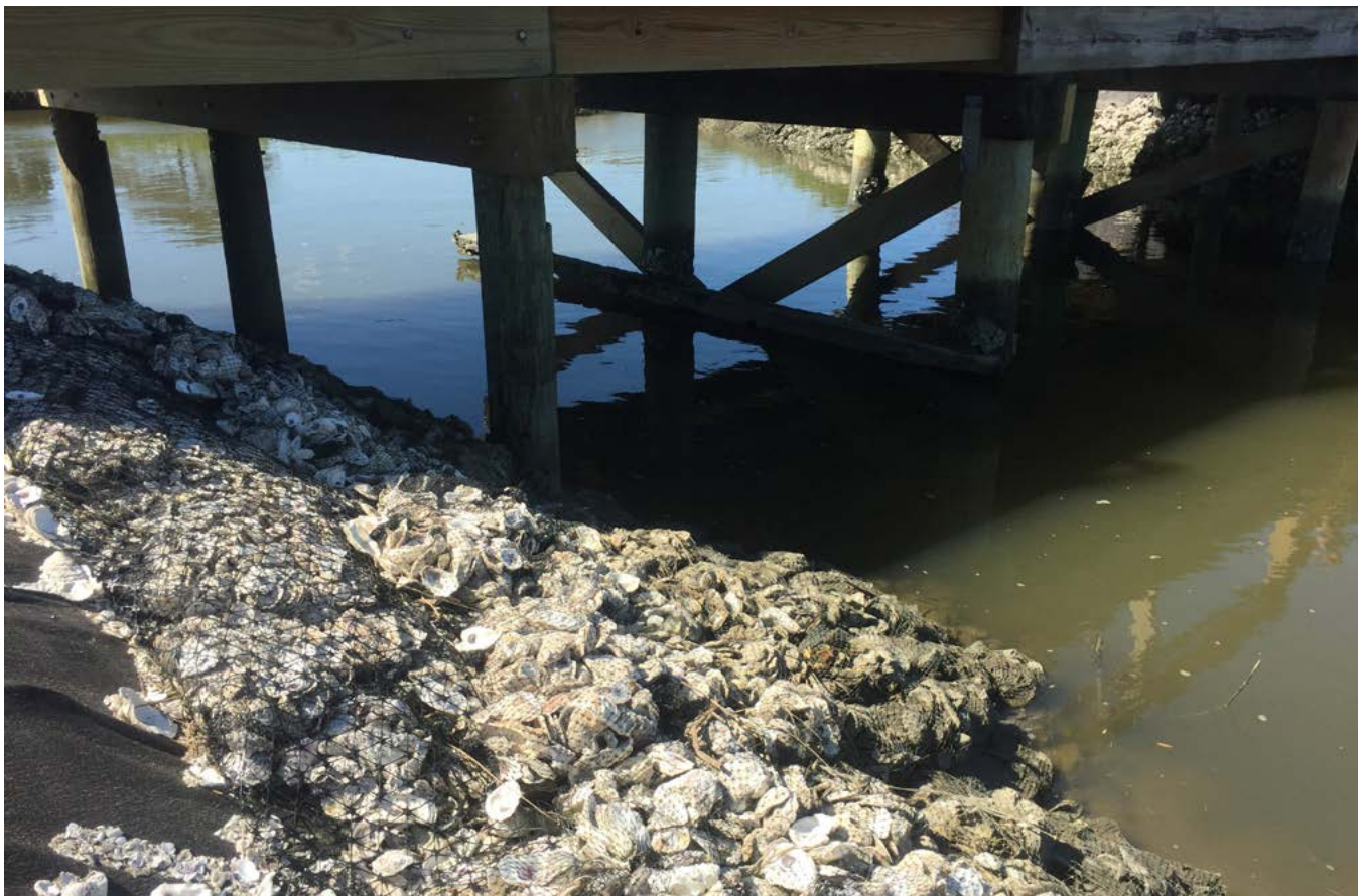
Tidal crossing incorporating bagged oyster shells for bank stabilization on Little St. Simons Island. Credit: Sara Gottlieb/TNC
