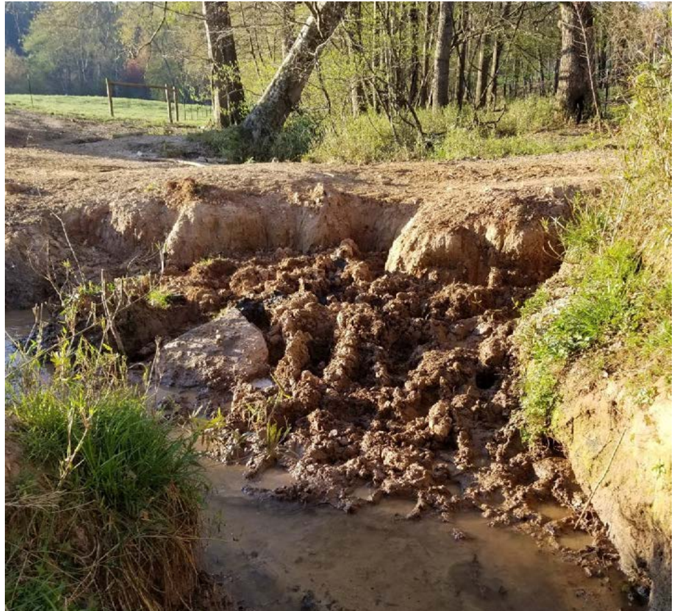
Before: A failed and undersized 24-inch round culvert that did not exclude livestock. Credit: Vance Crain/SARP
