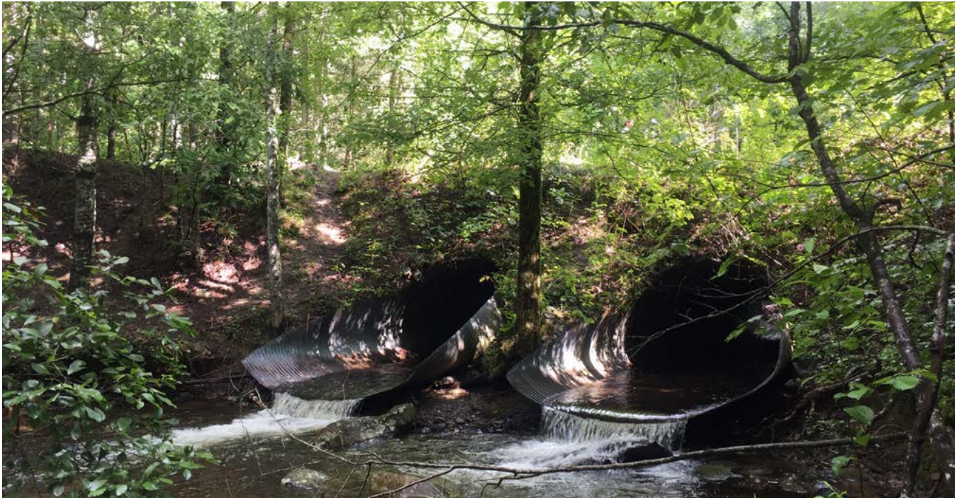
Before: Undersized and failing metal pipe culverts in 2017 on Mill Creek at Rocky Flats in the Chattahoochee National Forest. Credit: Sara Gottlieb/TNC
