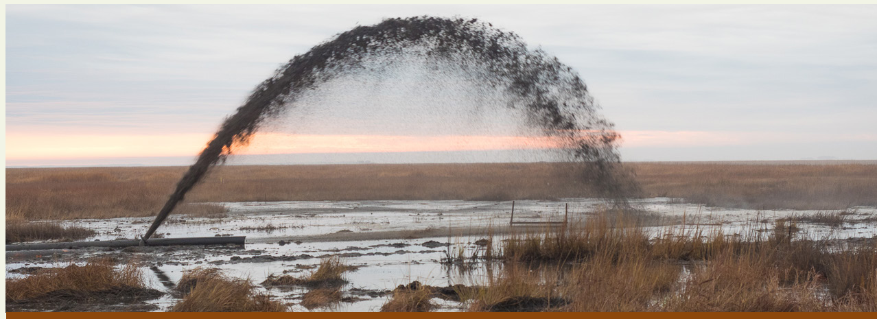
Thin layer deposition projects like this one at Blackwater NWR, spray sediments to compensate for its natural tendency to sink and the effects of sea-level rise. Dave Harp, Chesapeake Photos
