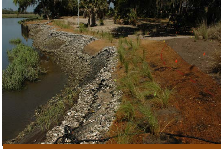
This living shoreline project constructed on Little St. Simons Island is a good example of a strategy to mitigate the effects of sea level rise and the negative effects of “hard” armoring shorelines. Todd Schneider
