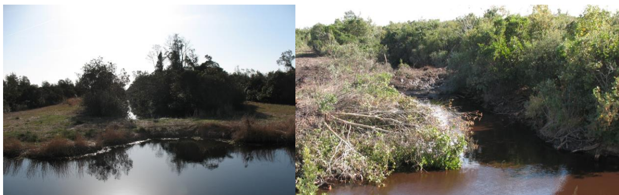
Figure A-13. Earthen plugs used to block water flow in a ditch/canal.
