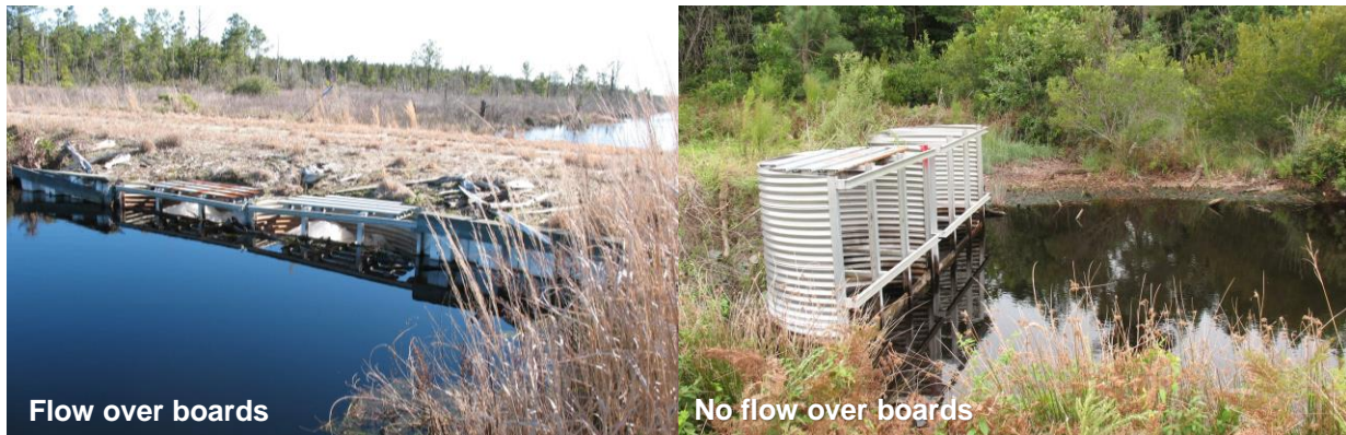
Figure A-12. Risers with water flow and with no flow over the top of the boards.
