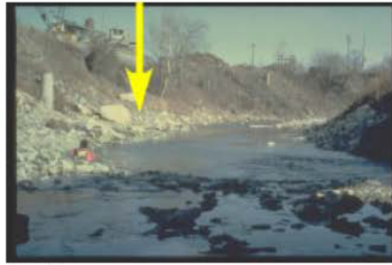
Poor Range (arrow highlighting unstable streambanks) (MD Save Our Streams)
