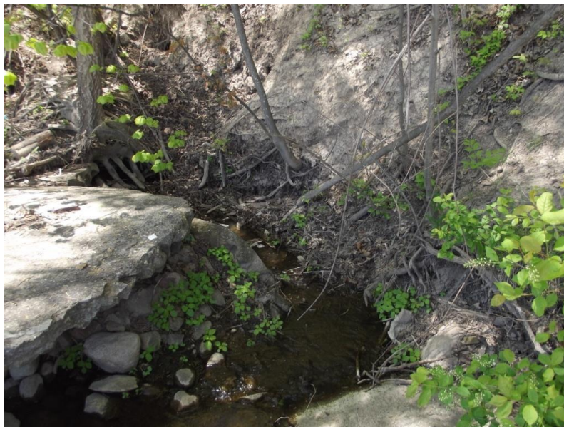
(Flow and erosion/slope failure at upstream end of west abutment wall) (Photo credit: Luke Trumble, MDEQ)
