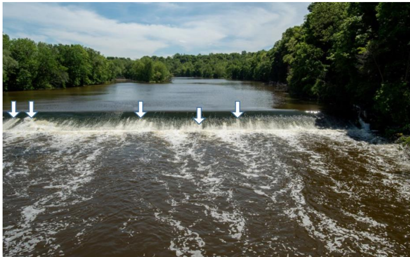
(Arrows indicating dam face fracture points and subsurface flow)
