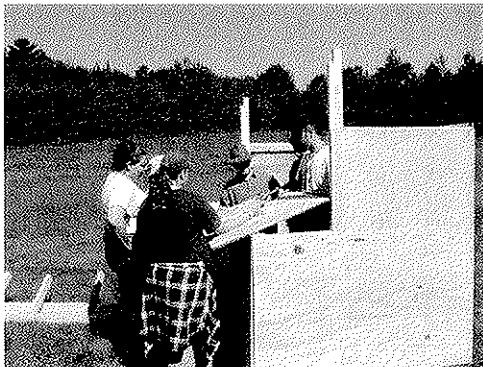
Duck Blinds. Last year's Youth Conservation Corps (YCC) constructed six observation blinds for the refuge. USFWS photo.
