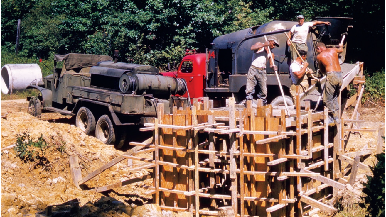
Works Progress Administration workers at Patuxent Research Refuge, Laurel, MD. Photo by Bureau of Biological Survey.
