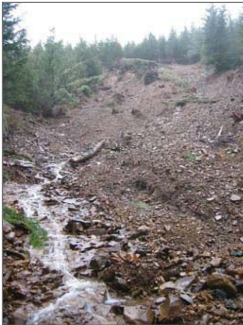
Figure 2. Landslide risk is generally moderate within the SWBCA although higher risks are associated with roads.
