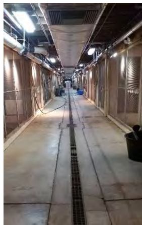
Indoor service area
