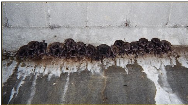
Photo 11: Bats roosting & associated staining
