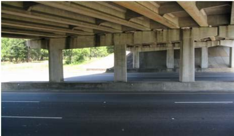
Photo 9: Staining on sides of pier caps
