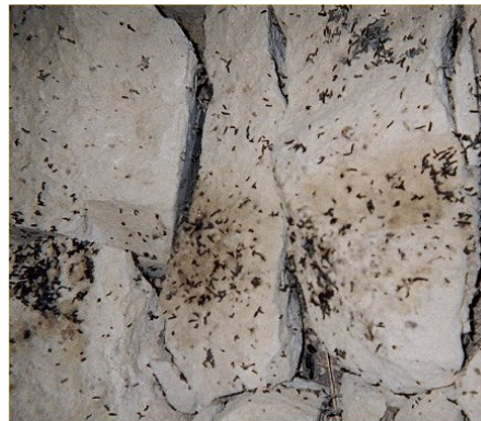
Photo 6: Bat Guano on Riprap
