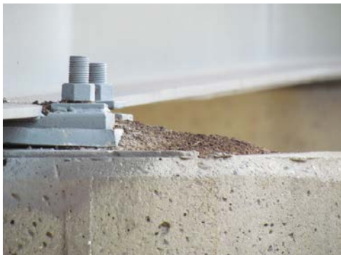
Photo 5: Guano deposit on pier, obscuring structural features.
