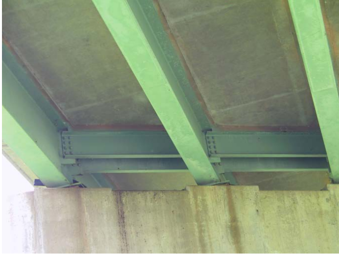
Photo 10: Guano staining on side of pier
