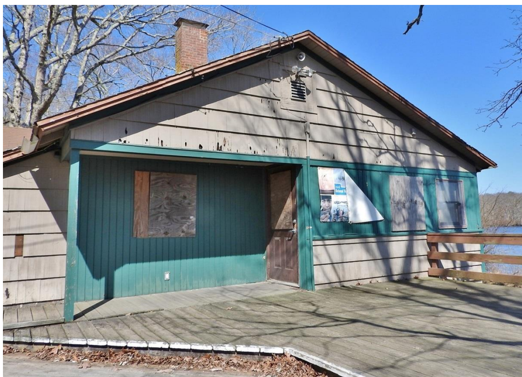
8. Facing northeast toward south elevation of main block. Full-height green siding installed in 1987 over location of original front door.
