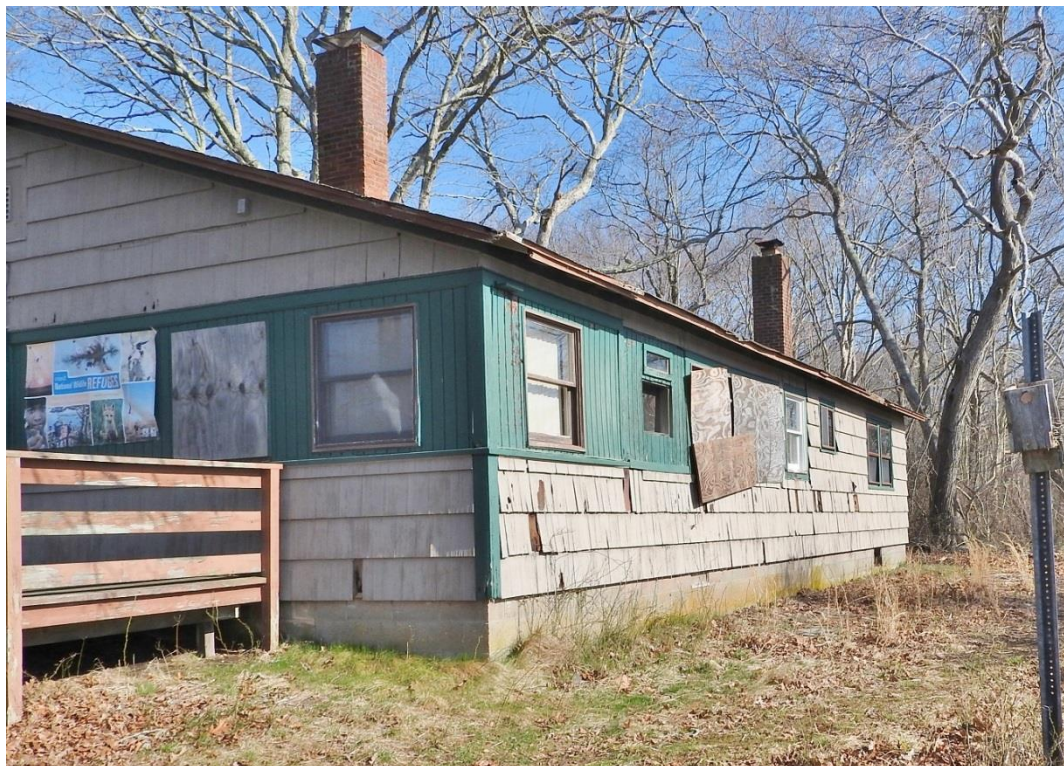
9. Facing northwest toward south and east elevations. Green siding installed in 1987 marks location of original recessed porch with jalousie windows.
