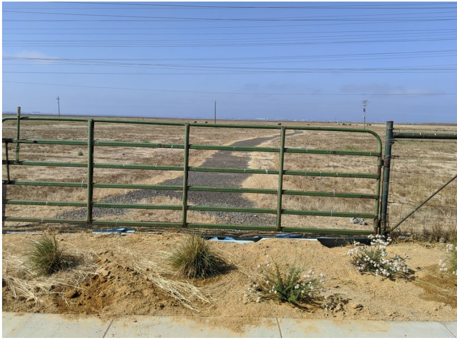
Figure 4. Photos of gate and pipe to be removed and existing access road to restore.
