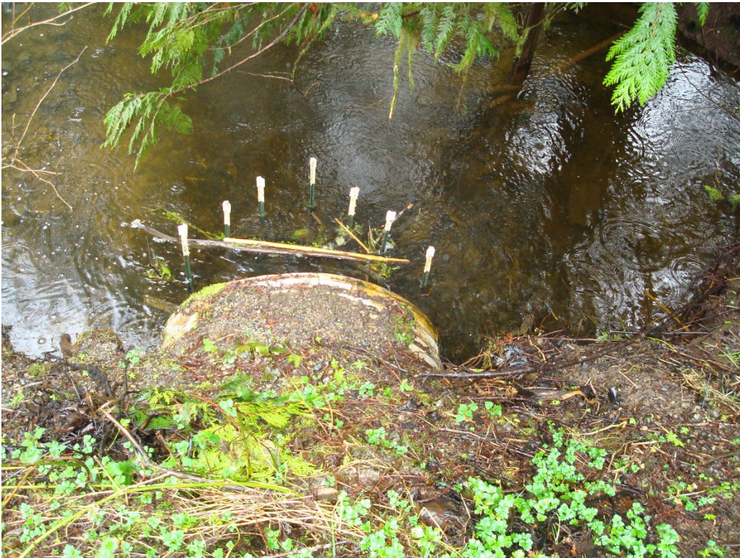
"T" posts at outfall prevents beavers from building inside
