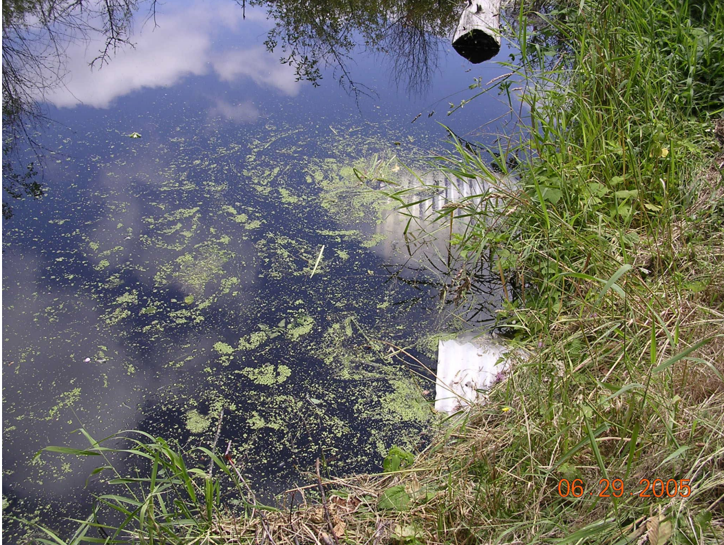
Submerged 4' diameter culverts with beaver dam built inside
