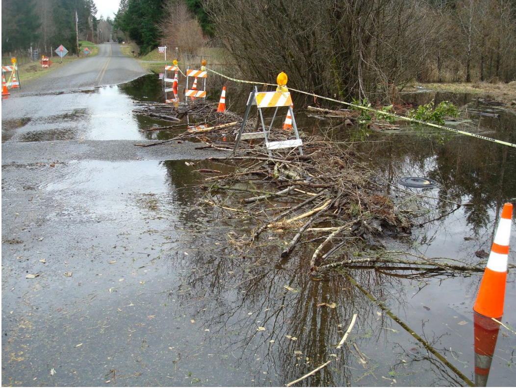
Roadside beaver dam – creates significant flooding and saturates road which leads to premature failure
