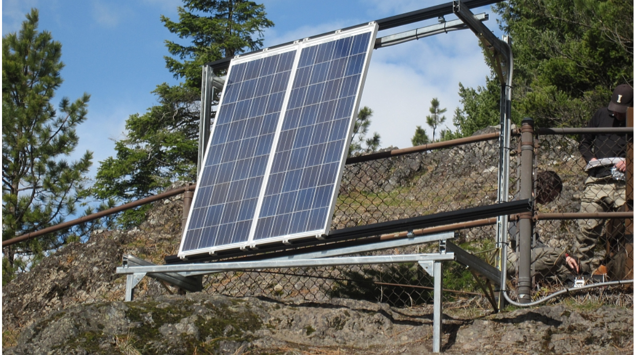
Figure 1. Solar panels installed to power the upper spillway and ladder antennae
