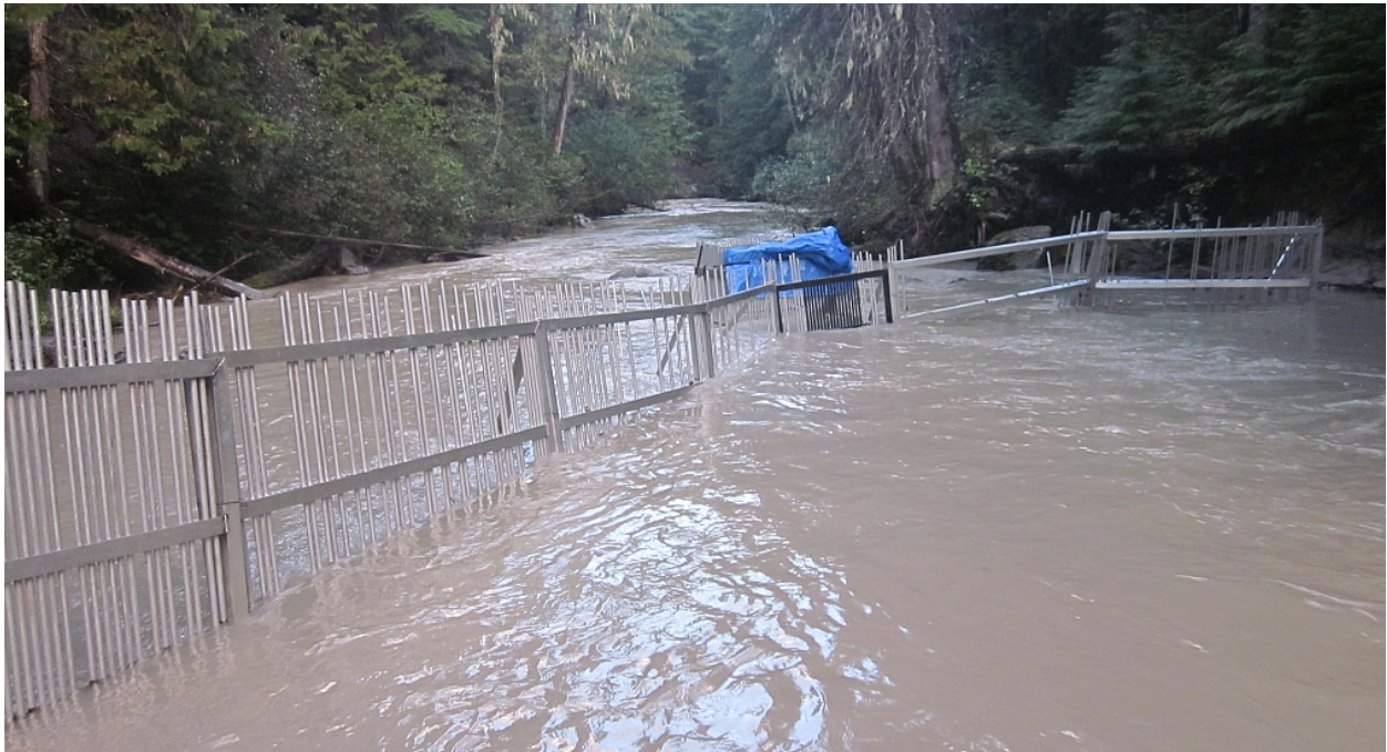
Figure 9. North Fork Tieton River fish trap after the high flow event on September 22, 2013 had partially collapsed the two weir panels on the right bank and weir pickets had been pulled to relieve pressure on the panels. The photo was taken the next day after the river had receded.
