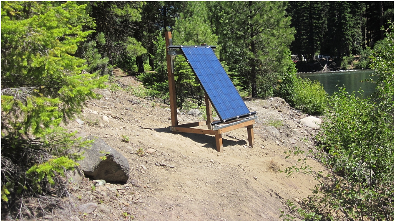
Figure 5. Solar panels installed to power the lower spillway antenna
