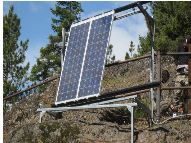
Solar panels at upper spillway/ladder site
