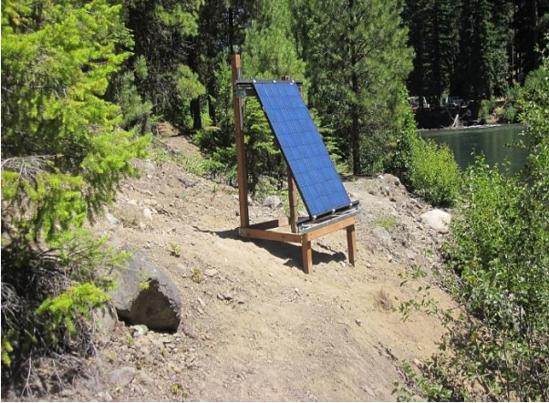
Solar panels at lower spillway site
