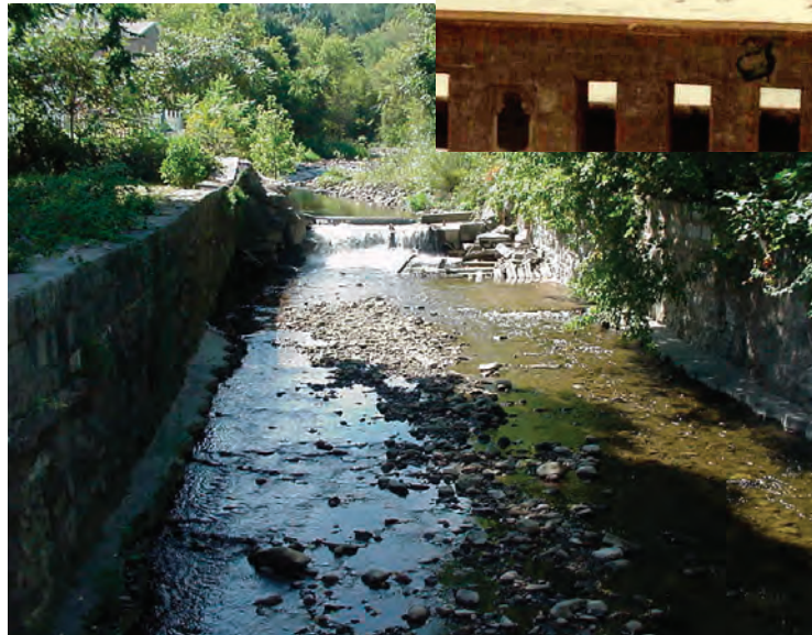
This channel was designed to carry a stream safely through a residential neighborhood. Unfortunately, the narrow channel and a low bridge clearance restrict the flow of ice, causing ice jams at this location. (Photographs courtesy of Herkimer-Oneida Counties Comprehensive Planning Program.)
