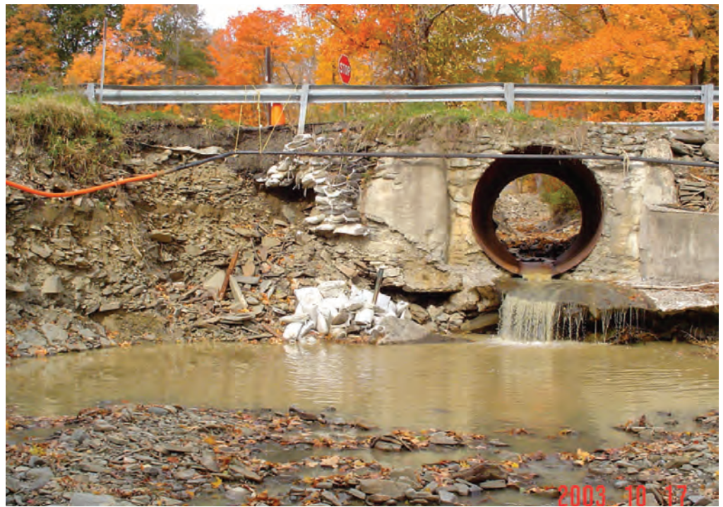
Water shooting out of this culvert has blown out the banks of the downstream channel. (Photograph by Mark Watts, Chemung County Soil and Water Conservation District.)
