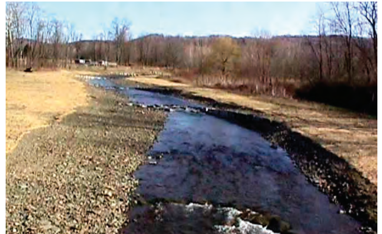
Rock structures have been placed in this stream to stabilize flow patterns and the channel. (Photograph by Mike Lovegreen, Bradford County Conservation District.)
