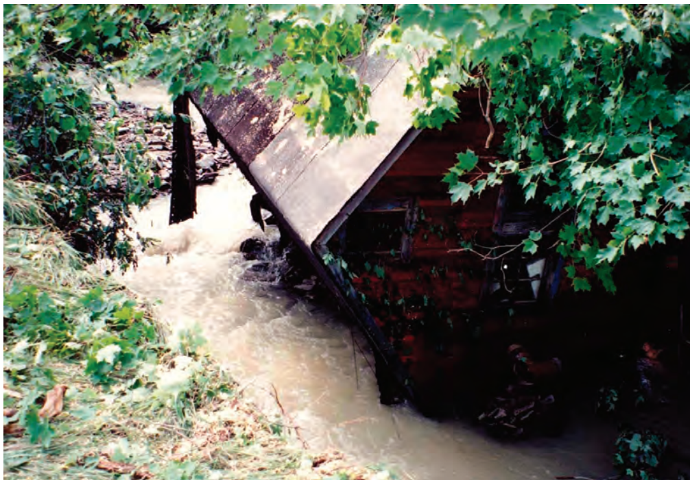
This house was completely undercut by streambank erosion and toppled into the stream. (Photograph by Mark Watts, Chemung County Soil and Water Conservation District.)
