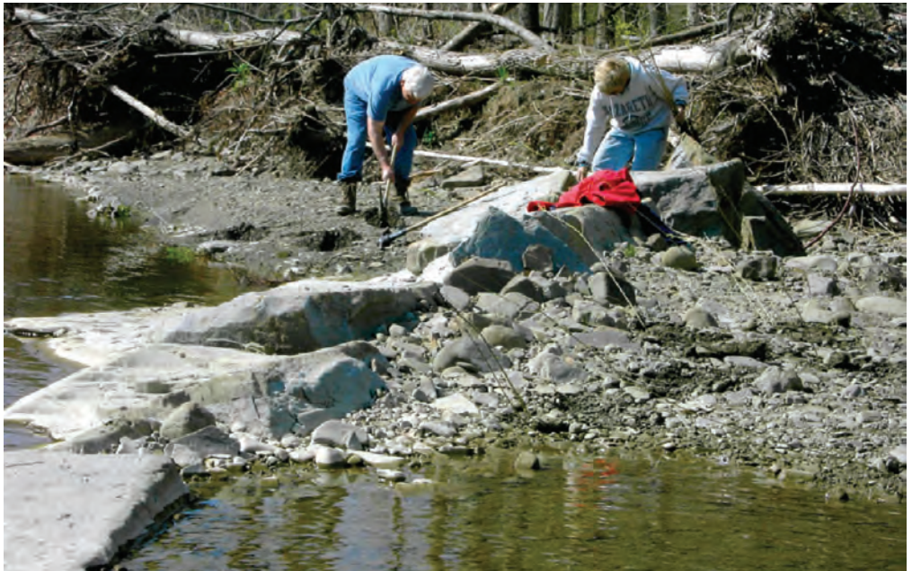
Volunteers are planting willows to stabilize a problem site in Steuben County. Once established, plants on the streambank and floodplain will dissipate energy and their roots will help stabilize the soil. (Photograph by Jeff DeMeritt, Meads Creek Watershed Citizens' Committee.)
