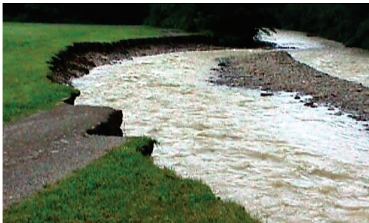
Flooding of this stream caused a washout extending 100 feet into the adjacent field. The site was restored by filling in the washed out area, stabilizing the bank with rock riprap, construction of two in-stream rock structures, and planting willows along the edge of the field. (Photographs courtesy of Steuben County Soil and Water Conservation District.)
