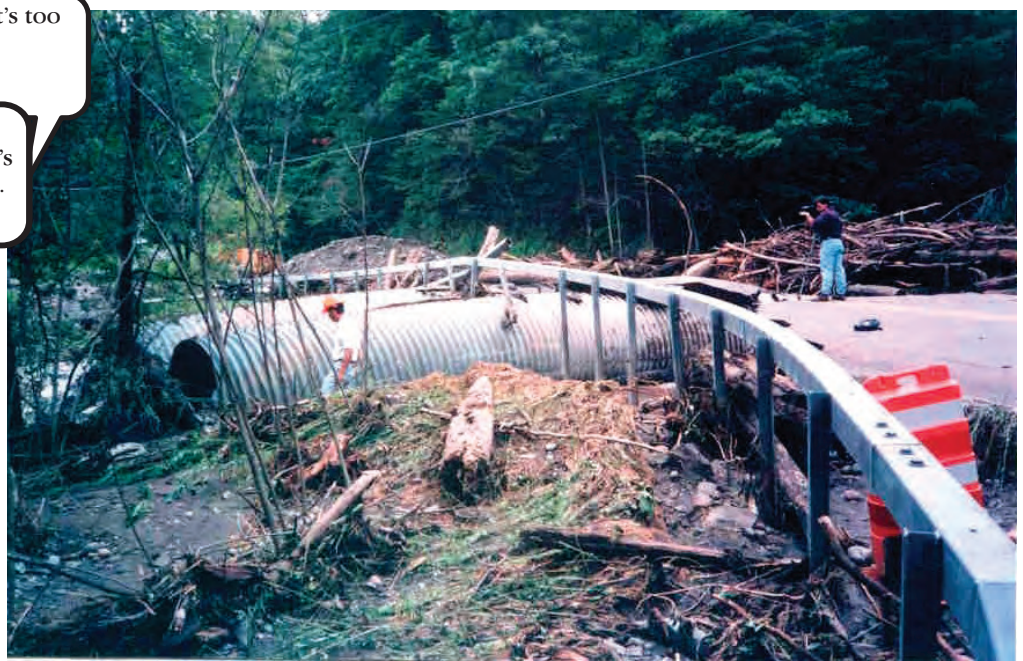
The design of some bridges and culvert imply not large enough to low for the high flow a d event. Wh fast moving floodwater i ociated cture, the bri e or culvert may be overtopped, d maged by washed out. oto- g aph rtesy of Herkimer-Oneida Cou sive Planni g Pro g
