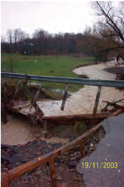
Floodplain flow was funneled under this narrow bridge, contributing to its collapse. (Photograph courtesy of Schuyler County Soil and Water Conservation District.)
