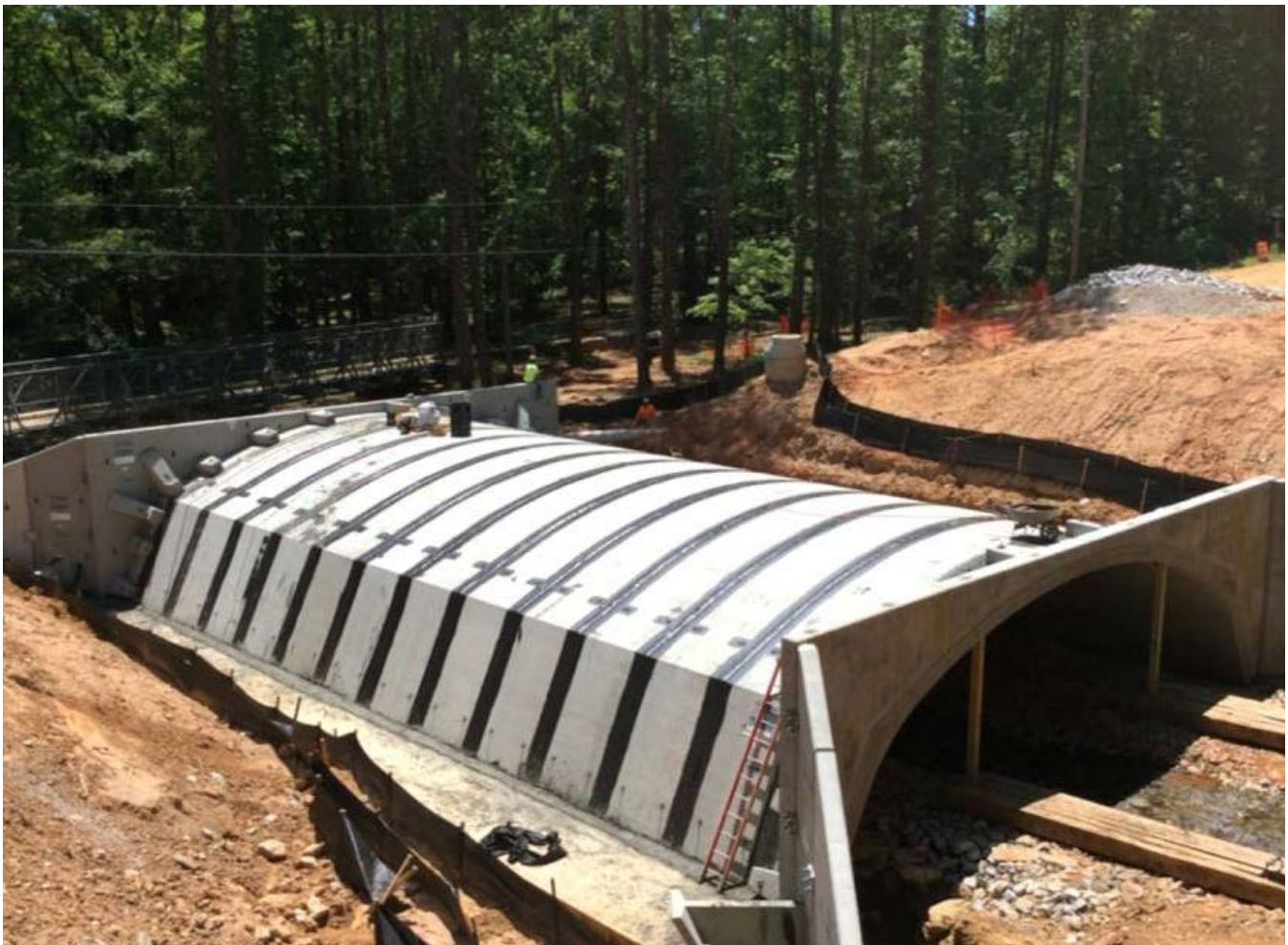
Concrete bottomless arch culvert being installed in Kedron Creek in Fayette County, funded by a SPLOST in 2017. Credit: Fayette County Road Dept.
