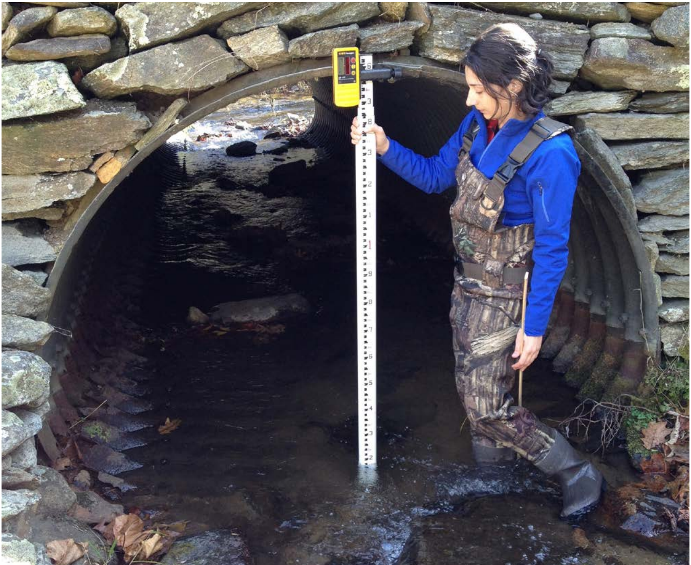
Field technician measures the height of a metal pipe culvert. Credit: Duncan Elkins/UGA
