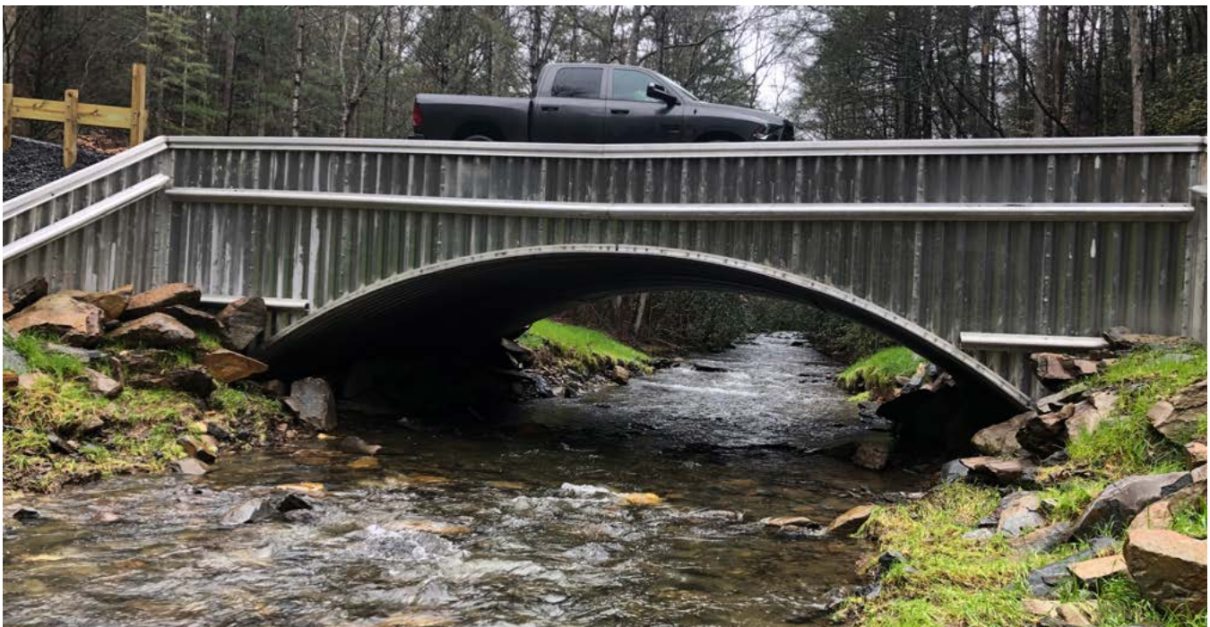
After: This open-bottom, prefabricated arch culvert replaced the failed Mill Creek stream crossing in 2019. Credit: Katie Owns/TNC
