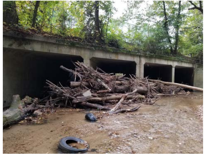
Box culverts clogged with woody debris and tires. Credit: Kelly Rudell/City of Atlanta DWM
