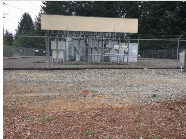
View west of substation.
