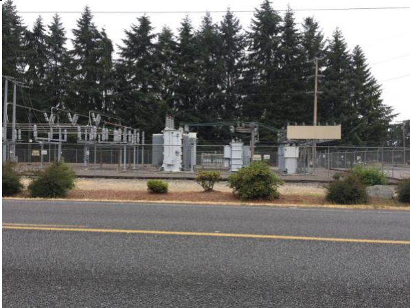
View north of Mullen Road and the substation
