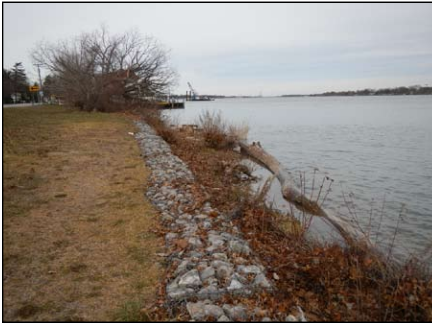
St. Clair River shoreline adjacent to Algonac State Park with gabion baskets.
