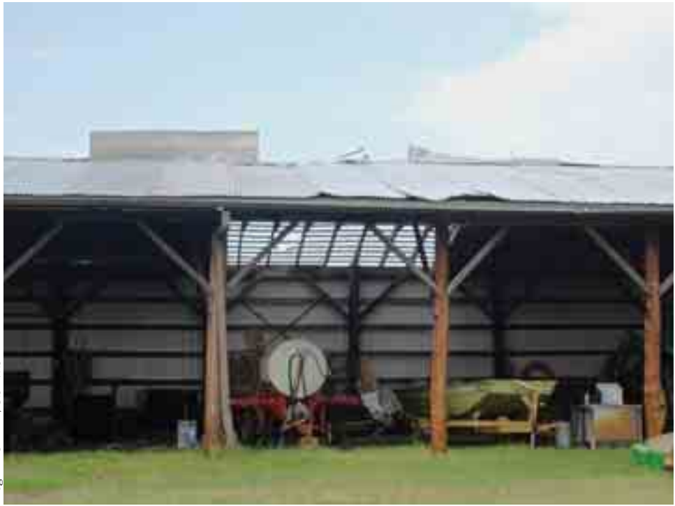
Pole barn after Hurricane Irene (August 2011)
