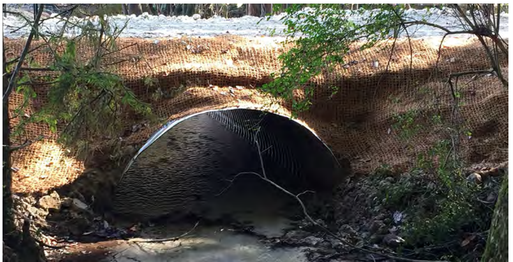
Installation of fish friendly culvert to benefit listed mussels in Chipola River tributary, Marianna, Florida, credit USFWS/Chris Metcalf.
