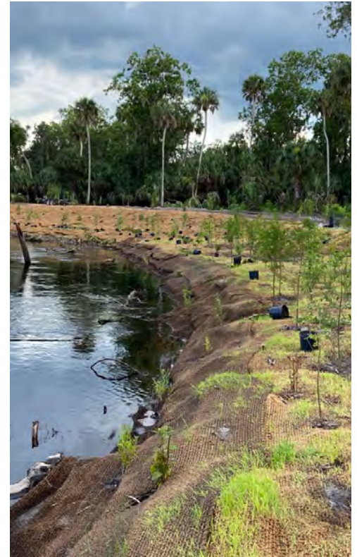
Streambank stabilization to benefit the threatened Florida manatee in the Peace River, Zolfo Springs, Florida, credit USFWS/Chris Metcalf.
