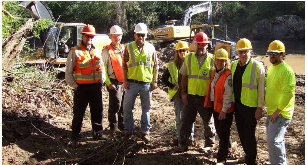
Partners Biologist Laura Fogo and members of the Service's Aquatic Habitat Restoration Team on site during the removal of the Troy Dam in Montgomery County, NC, credit: USFWS.
