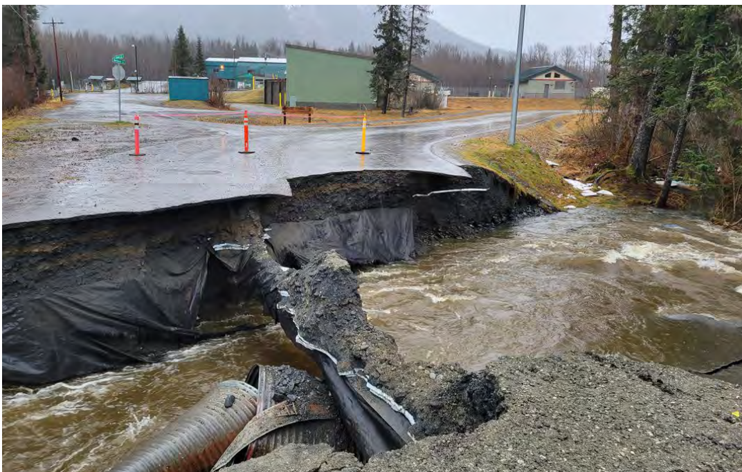
Photo: Heavy rains, flooding, and a washed out culvert in Girdwood, October 2021. (Dave Leval, KTUU)
