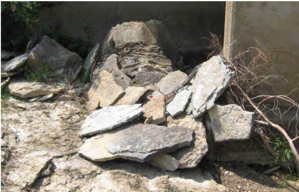
Fig. 6. Rock slabs pushed against a bridge by the May 2010 flood.
