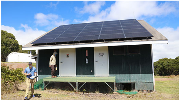
Photo-Voltaic (P-V) Power Building
