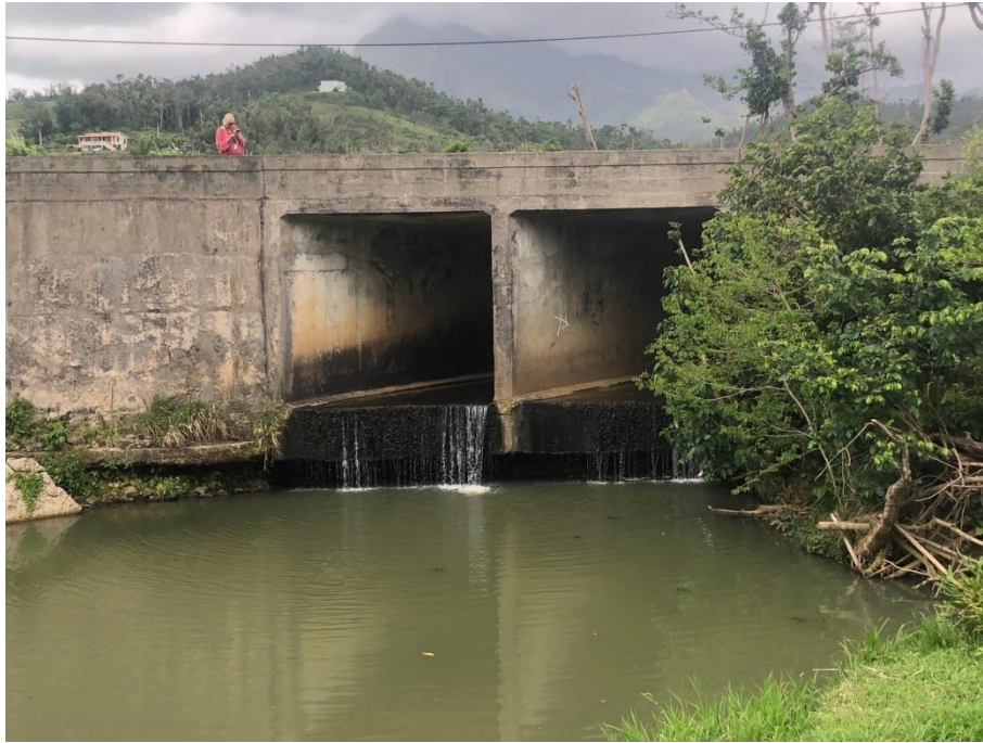
Figure 5. Poor design has resulted in scour and degradation below culvert and obstruction to fish passage.
