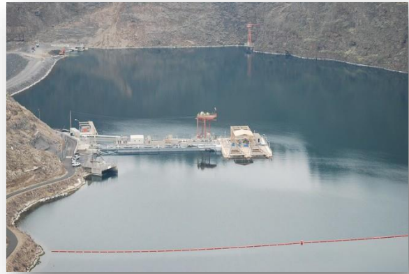
Figure 158: Construction sequence of the new selective water withdrawal and fish collection facility at Round Butte Dam, Lake Billy Chinook, Deschutes River, Madras, Oregon. Photo by Scott Carlon, NOAA Fisheries
