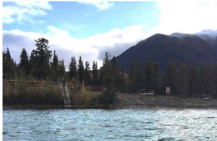
The left side of the photo shows a completed section of the Kenai River project with re-vegetation and completed stairway.
