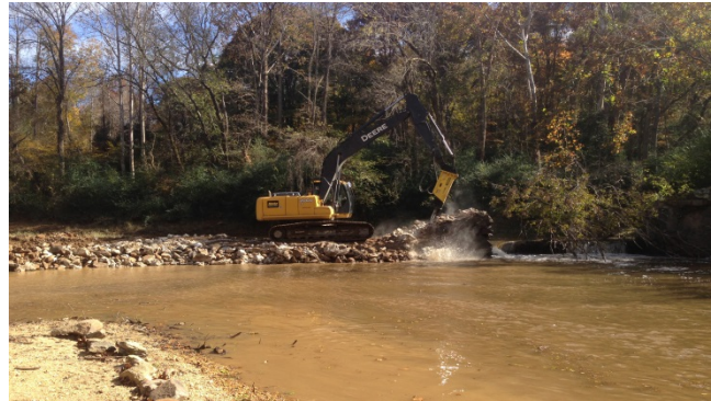
The West Fork Dam removal and fish passage project improved public safety, reduced landowner liability, and reconnected over 950 miles of streams and tributaries. Credit: USFWS
