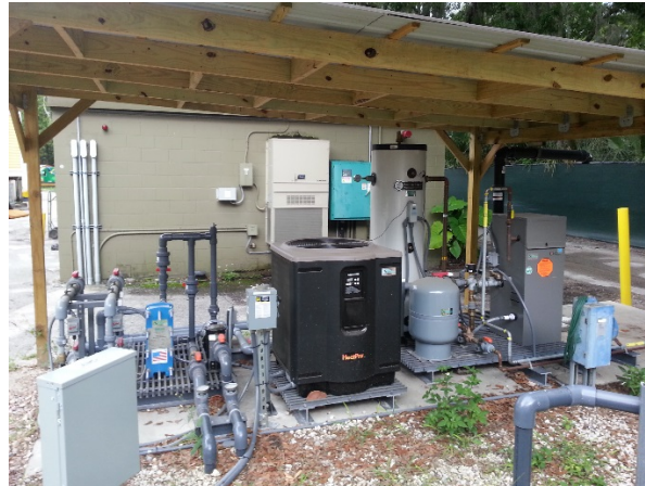
Image 9: Heater and chiller unit for medical pool 1
