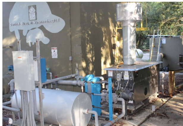
Image 10: Heating unit for the recovery pools and medical pools 2 and 3
