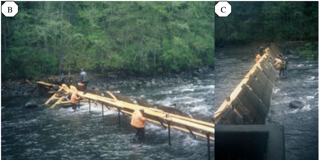
Figure 1. (A) Aerial photograph of White Salmon Ponds, a historical brood stock collection facility operated by Spring Creek National Fish Hatchery located at river mile 1.4 on the White Salmon River. (B, C) Pictures of Spring Creek NFH staff constructing the historical picket weir that would block upstream migration of Lower Columbia River Fall Chinook salmon adults for redirection in the White Salmon Ponds. Returning adults were trapped and collected to supply the annual production of Spring Creek NFH production through the late 1970's, and intermittently thereafter. Adult collections have not occurred at the site since the early 1990's. Photos courtesy of PacifiCorp.
