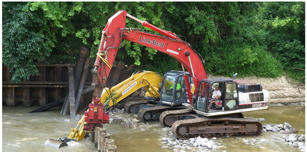
The PFW program partnered with the private landowner and multiple other partners including the Service's Fisheries and Aquatic Habitat Restoration Team to remove the Livingston Dam on the Sucarnoochee River in western Alabama. Removal of this dam improved habitat in a designated segment of Critical Habitat for four federally protected mussels and two at-risk species. Over 600 miles of river and tributaries were re-opened for fish passage and the river now flows free for its entire length, credit: Eric Spadgenski.
