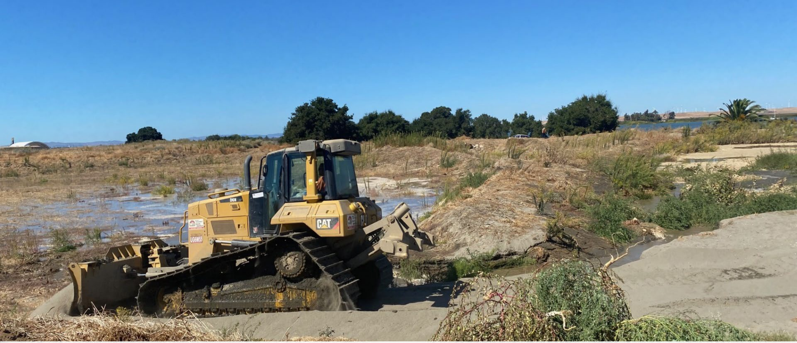
US Army Corps and Port of Stockton Contractors preparing site for reception of new sand material with refuge staff guidance. They arrived September 25 th , 2023 and finished October 3 rd , 2023.
