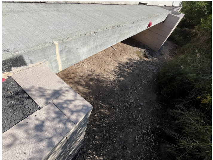
Ocelot Crossing Culvert at Laguna Atascosa NWR. Source: Nate Begay, FWS
