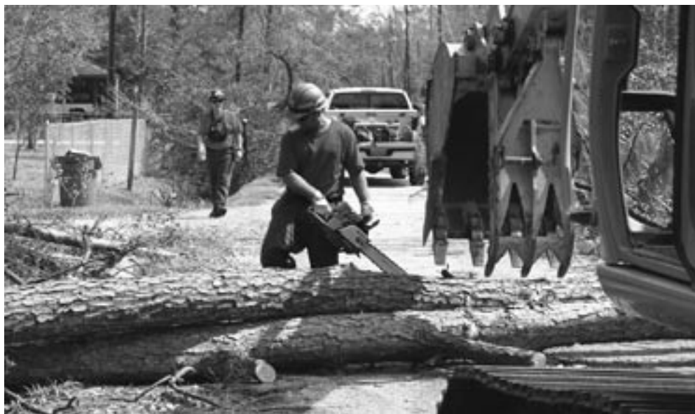
Road clearing was often necessary for Service crews dispatched to provide post-storm assistance.
