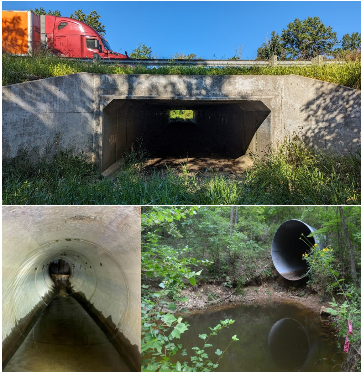
FIGURE 8. Representative culvert structures of various types, including a box culvert in Indiana (top; photo by USFWS); a round, concrete pipe culvert design in Georgia (bottom left; photo provided by Georgia Department of Natural Resources); and a corrugated metal pipe culvert design in Missouri (bottom right; photo provided by L. Droppelman).
