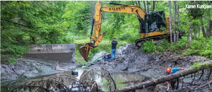
The demolition of one of the three dams removed on Frost Gully Brook.
