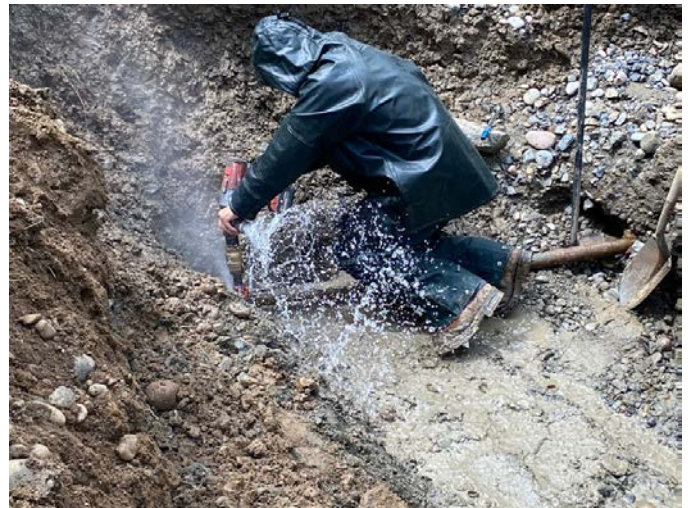
TRYING TO STOP THE LEAK
