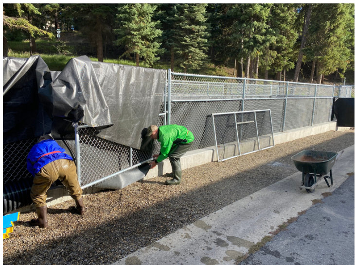
TEMPORARY SHADE STRUCTURE
