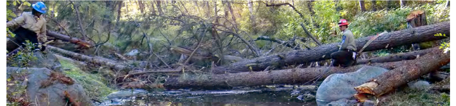
PFW is a leader within the Department of Interior in implementing Nature-Based Solutions by delivering conservation projects such as stream restoration, culvert replacement, fish passage, fuel management, pollinator gardens and reforestation. Photos ©USFWS.
