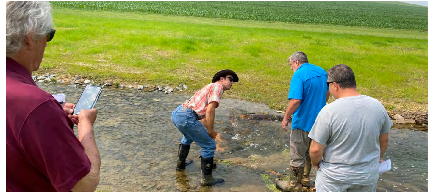
USFWS, Unique Excavating and Pheasants Forever staff, working to restore Indian Spring Run and an adjacent cold-water tributary. ©USFWS.
