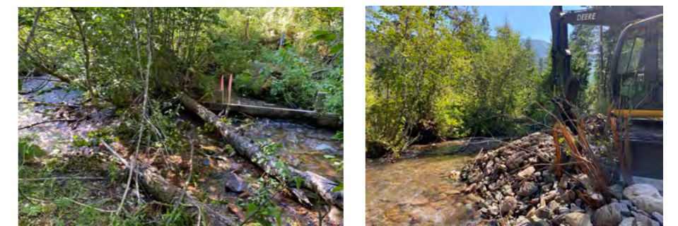
A view of the unscreened irrigation ditch, looking downstream (left), The formerly unscreened ditch was plugged with on-site sediments, backed by geotextile fabric, and reinforced with willow transplants (right). ©USFWS.
