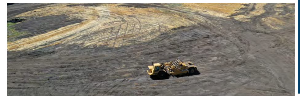
Wetland construction with refuge owned equipment operated by PFW staff. © Matt Blakeley-Smith.
