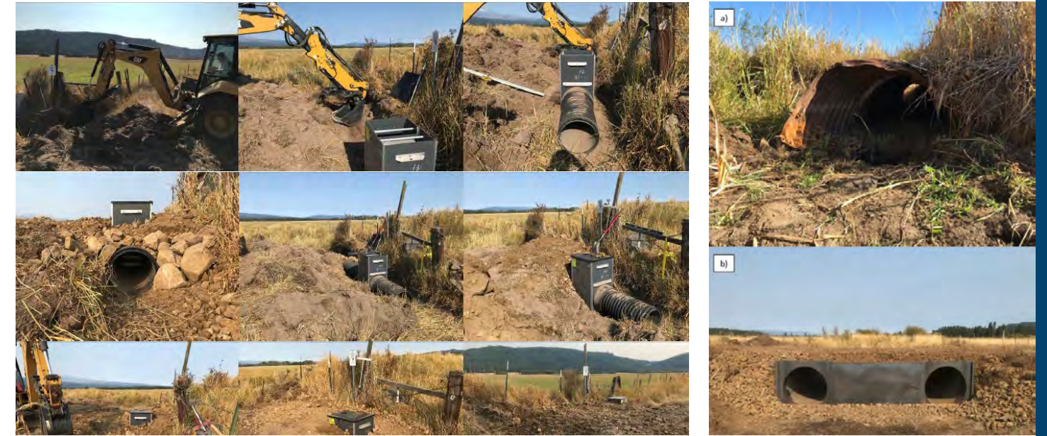
Lef to right: Compilation of photos documenting water control infrastructure installation in Glenwood Valley, Washington. Photo collage starts with site prep at the top left, reads left to right, ending with final install photo bottom right) Right Before (a) and after (b) photos of water control infrastructure at OK Ranch. ©USFWS
