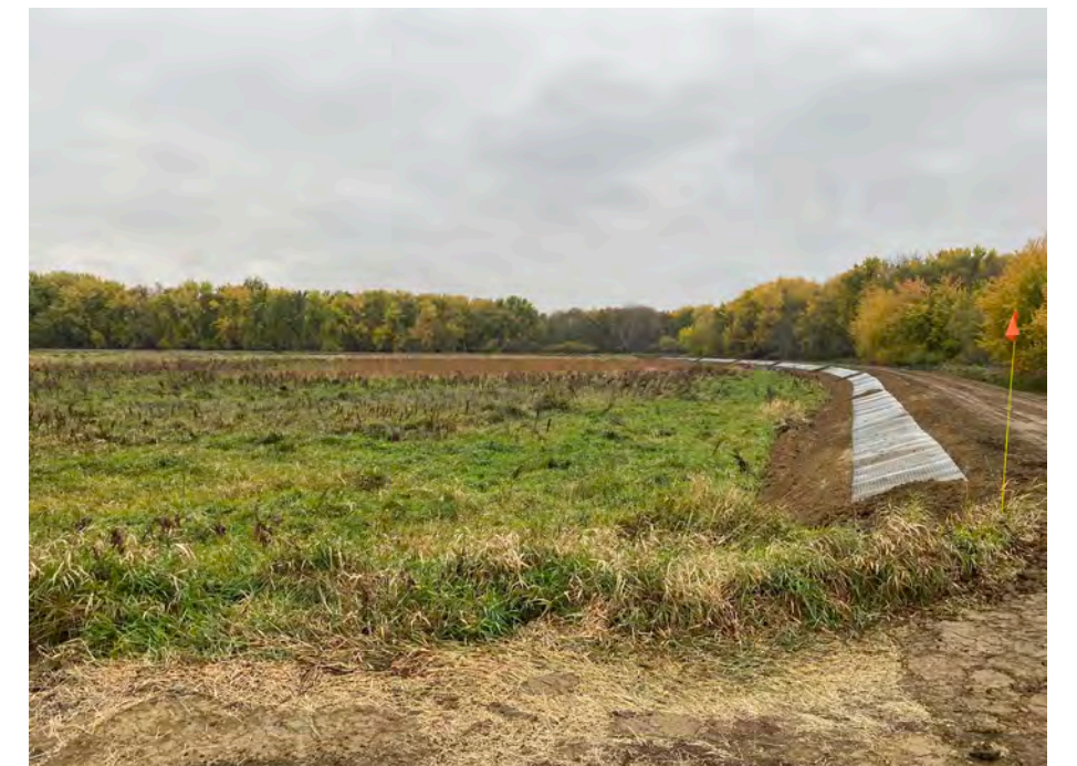
This project reshaped the dike (wider top and flatter side slopes), armored the dike with riprap in critical areas, installed rat wire to reduce rodent damage to the dike, and cleaned out the WCS to ensure they are functional. ©USFWS
