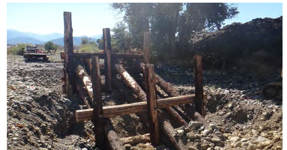
Large wood structure during construction. Vertical posts are buried into the river bed and the horizontal posts are bolted to the vertical posts. Large boulders are placed around horizontal posts for ballast and in front of the structure for scour protection. River bed material excavated for the placement of the vertical posts is used to fill in the interstitial spaces within the wood structure.
