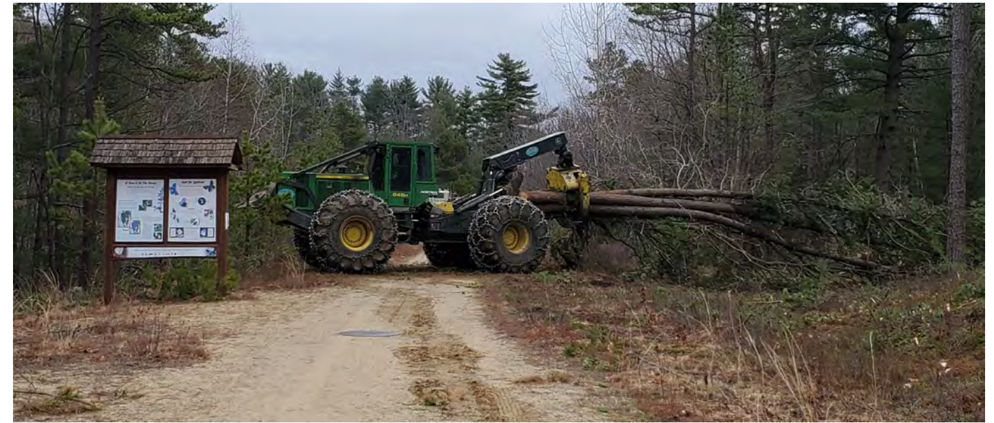
Skidding / tree removal at project site to benefit the Karner Blue Butterfly. ©USFWS
