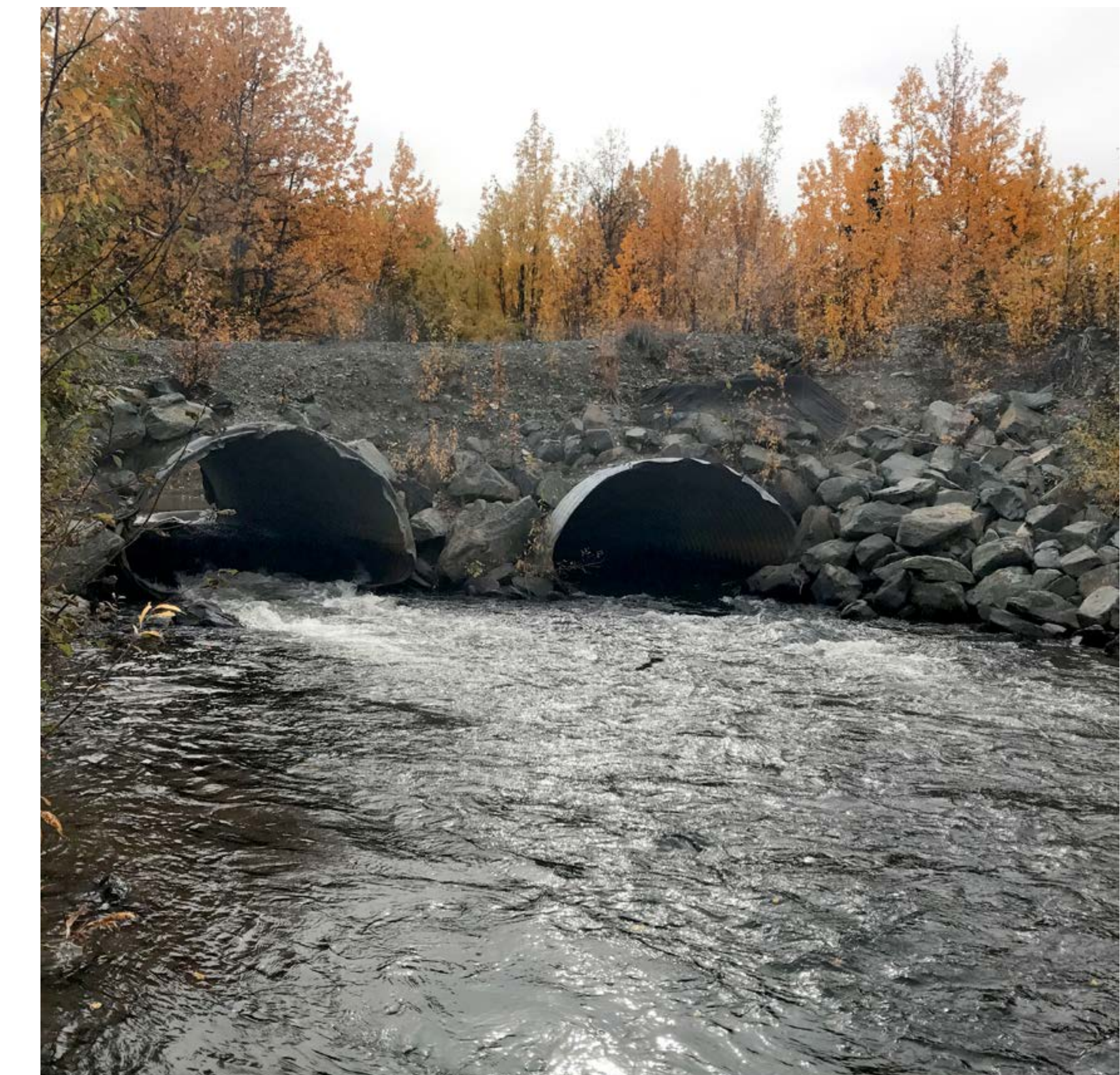
Two undersized culverts on the Little Tonsina River in Alaska. Photo credit: USFWS
