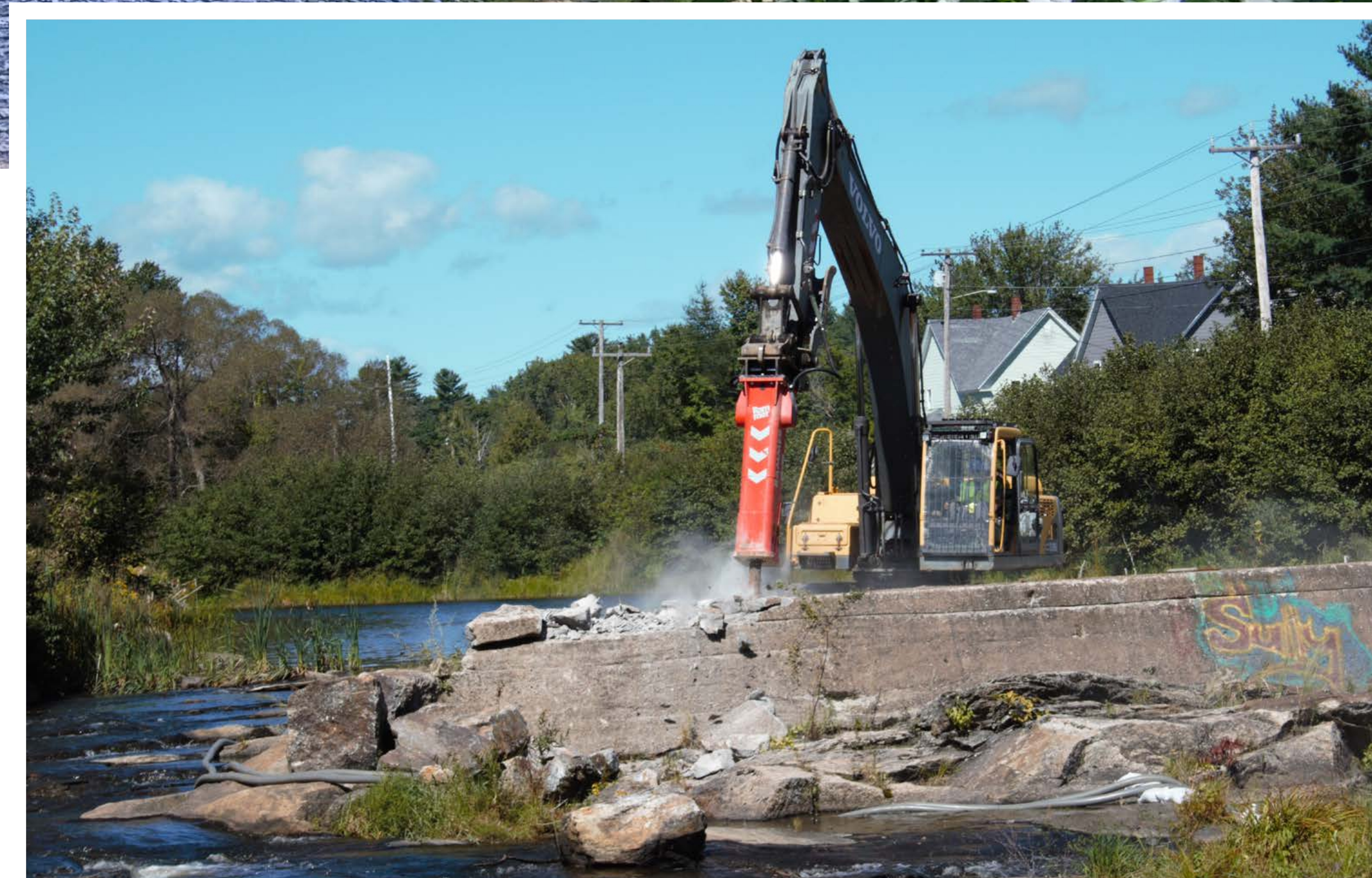
Construction crews demolishing Town Dam on the Sabattus River in Maine. Photo credit: Catherine Birmingham/ASF
