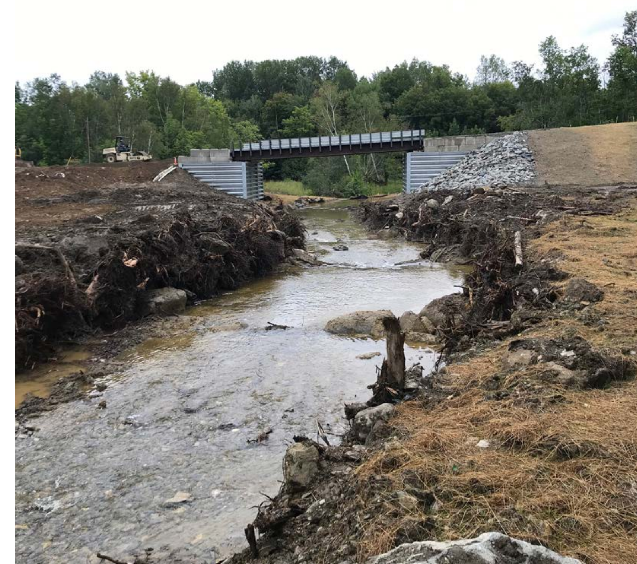
Moose Brook finished bridge in Houlton, Maine. Photo courtesy of Sue Young/Houlton Band of Maliseet Indians
