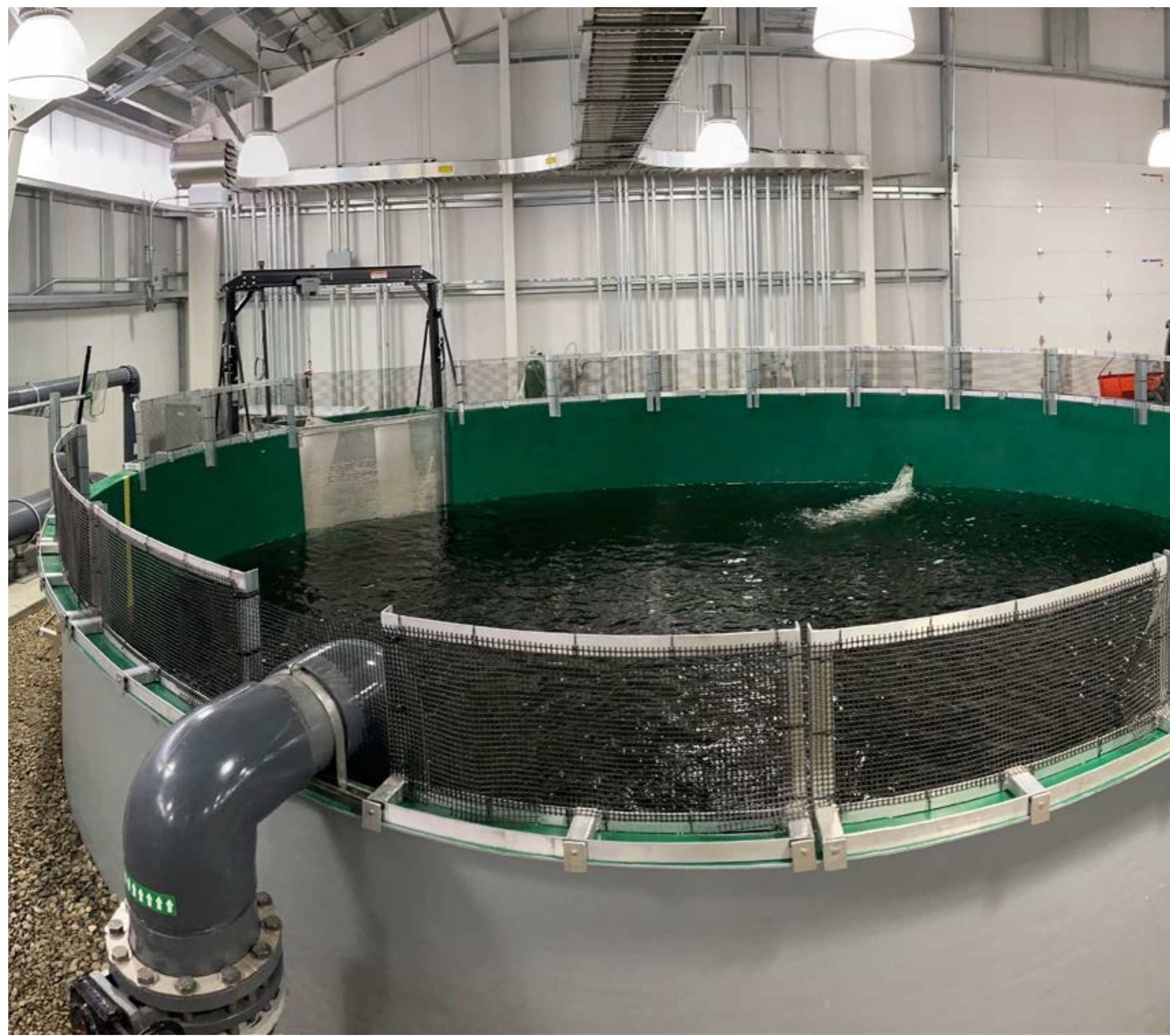
Circular tanks used in the PRAS system. Photo credit: USFWS
