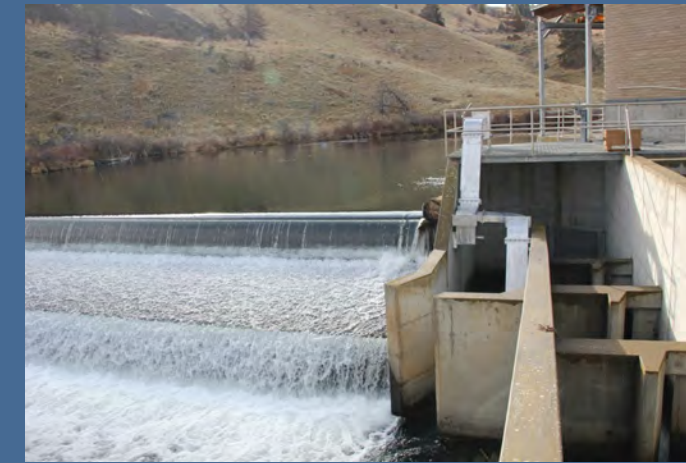
Warm Springs National Fish Hatchery's energy network received several upgrades in 2018-2019. The hatchery also installed at Lamprey Passage System in 2018 that helps adult Pacific Lamprey access to the Upper Warm Springs River. Photo: Terry Freije/USFWS
