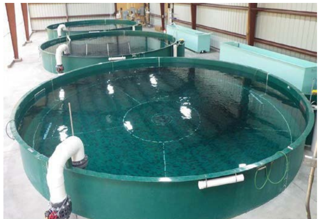
A circular tank water re-use system at Hagerman NFH. How do we calculate FI in re-use systems?
