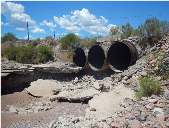
Photo 20. View of culvert system that is a barrier to upstream fish passage at East del Chi Dr crossing, 7/28/20. Each culvert is approximately 6 ft in diameter.
